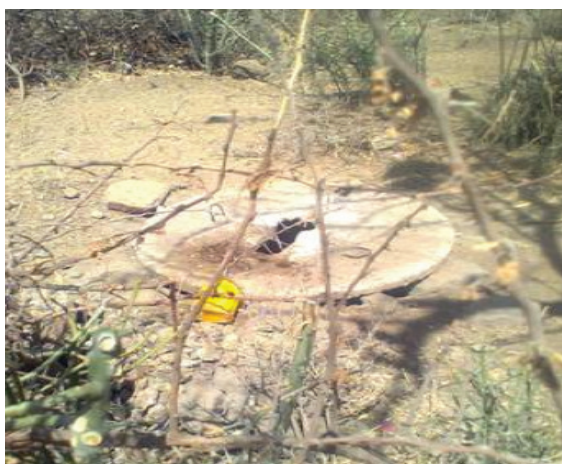
Latrine in use but no superstructure
