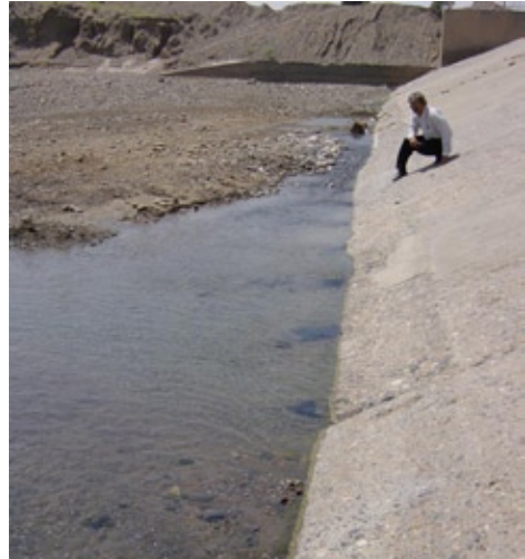
Figure 3: Water emerging from weepholes
