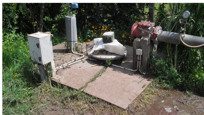
Scope for improving well head protection
