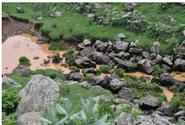
The foundation conditions are very good and the bed rock is visible in both embankments and the river bed.
